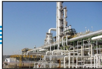
Oil Refinery Pipelines Plants
