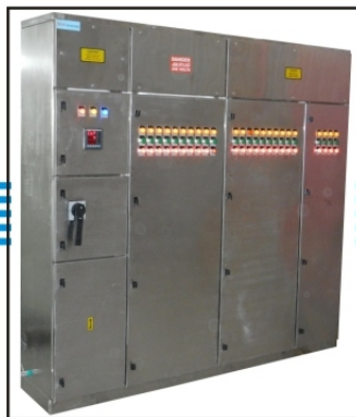
Electricals Panel Bord Plant
